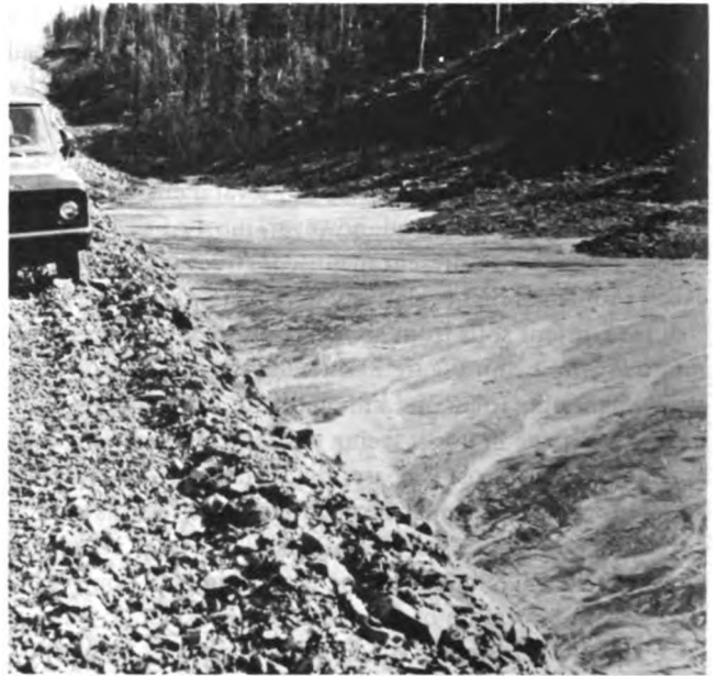
FIGURE 5 Backslope erosion into parallel ditch, 31.6 km, 26 June 1970.
