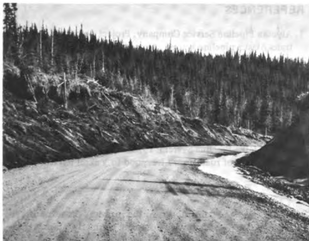
FIGURE 14 Additional slumping of backslope, 32.6 km, 28 May 1971.
