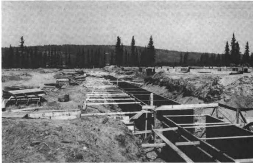
Stop 24. Concrete utilidor under construction at Fort Wainwright near Fairbanks. This area is on the Chena River floodplain and is underlain by perennially frozen sand and gravel with low ice content. (Photograph 139 by T.L. Pévé, July 16, 1947)
