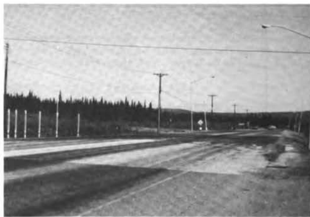
Stop 2. Note in the distance, tilting of the light standards and signs and telephone poles along both sides of the road which indicates thawing of the ice-rich permafrost with associated subsidence of the ground. (Photograph 25443 by T.L. Pévé, May 15, 1983.)
