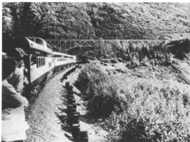
Train crossing active segment of Moody Landslide. Piles along shoulder were installed to help control downslope movement of the roadbed.
