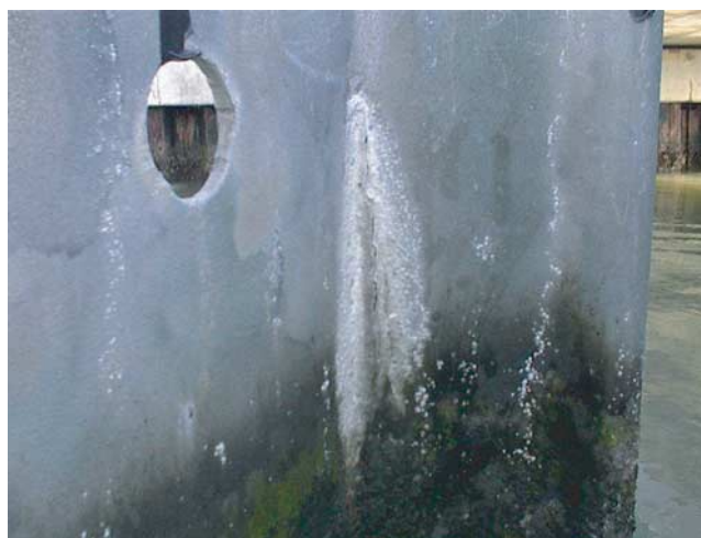
Figure 1. Thermal spray aluminum (99.5 percent) coating in seawater after 2 years exposure.
