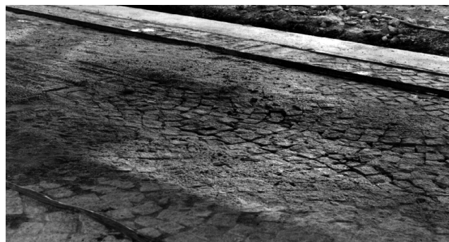
FIGURE 17 Failure of block pavers after 9,000 cycles of 40-kN loading. Note the amount of sand that has been pumped from under the granite blocks (Sharp 2001).
