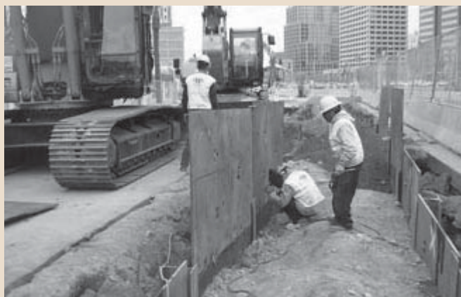
A work crew welds plates before driving them into the ground during LRT construction in Phoenix, December 2005.
