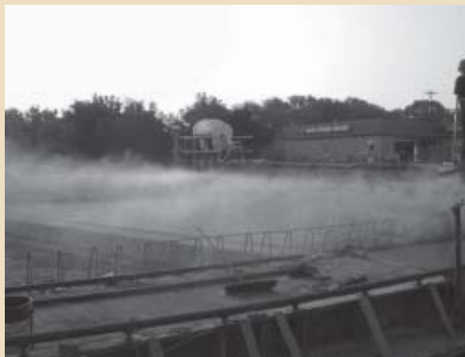
In unfavorable weather conditions, fogging of concrete—here, during placement on an I-70 bridge—reduces cracking on new decks.
