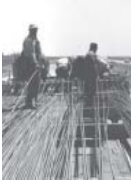
The original Interstate construction required durable materials (above). The next phase also may call for a “wired” system equipped with high-tech intelligent transportation devices.
