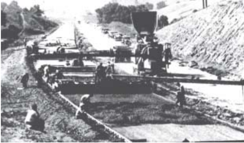
Construction on the Pennsylvania Turnpike in the late 1930s. The Interstate precursor raised U.S. geometric and design standards for highways.
