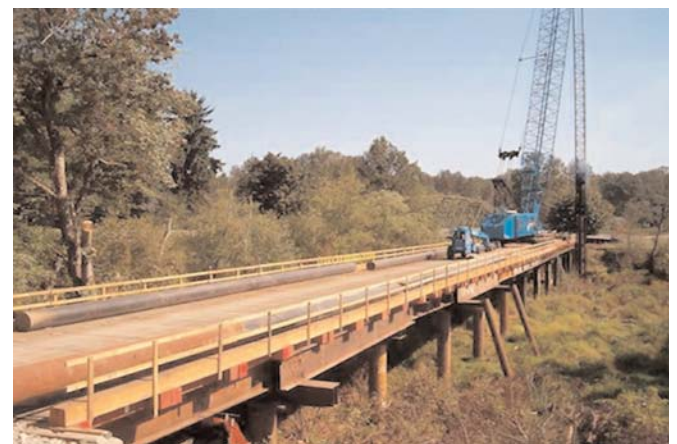
Figure 2 Temporary contractor designed trestle bridge used for construction of Tolt bridge, King County, WA.
