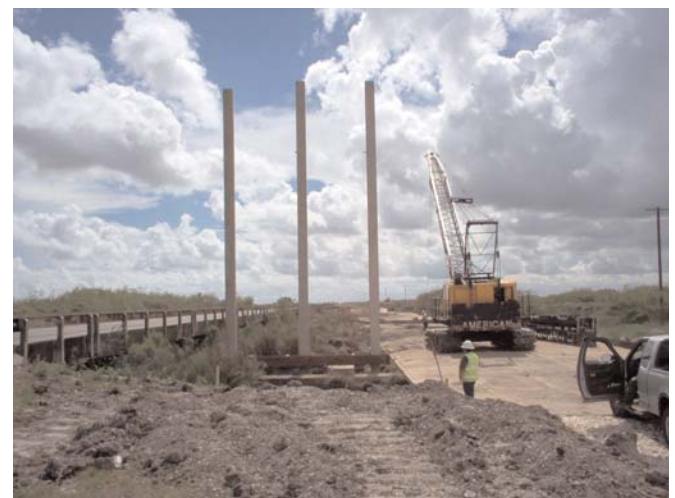
Figure 6 A composite mat system provides construction equipment access at the Cavasso Creek bridge project in Aransas County, TX.
