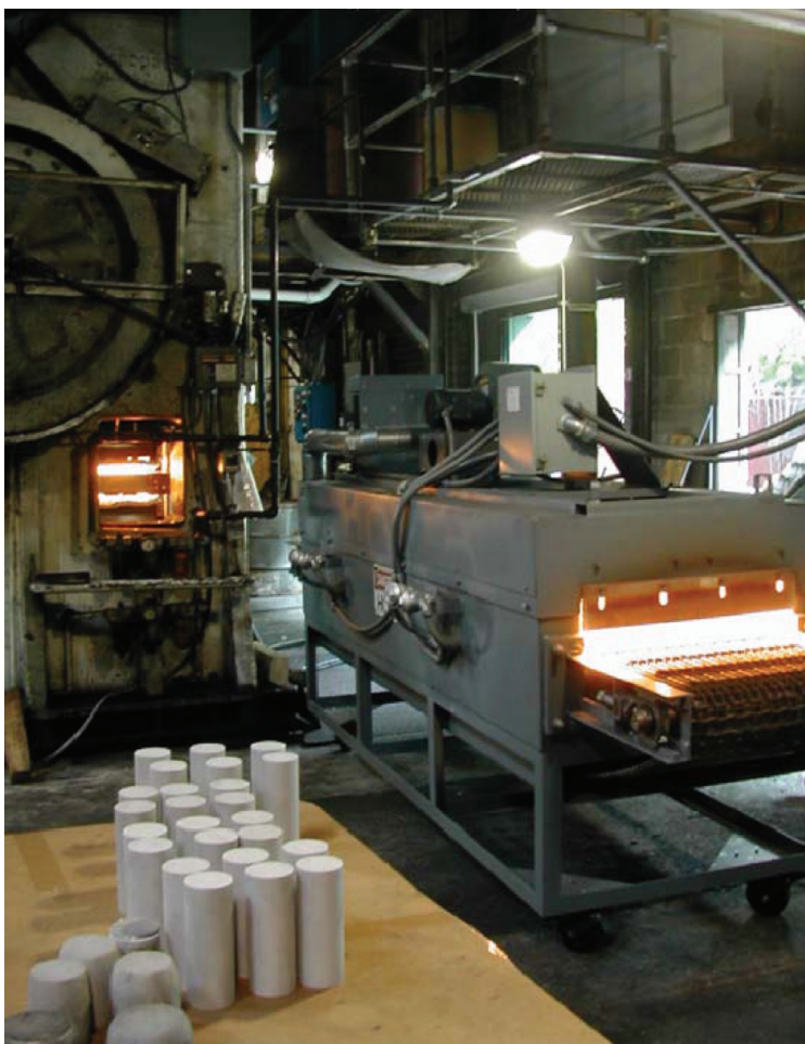
FIGURE 4.8 Continuous-belt infrared furnace for high-performance aluminum forgings. Testing of this system at Queen City Forging Company confirmed that it is more than three times more energy-efficient than current convection furnaces in preheating aluminum billets. It also provides grain refinement that enhances fatigue properties. Infrared preheated and forged components have been shown to last two times longer than conventionally preheated forgings. Source: DOE/EERE, 2005.
