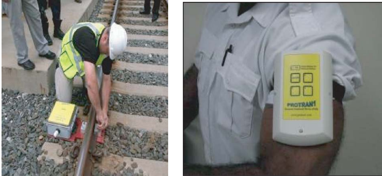
FIGURE 14 Examples of portable warning devices. Portable train detection device being installed on ROW (left); employee wearing PAD used by MBTA and MTA (right) (Courtesy: MBTA).
