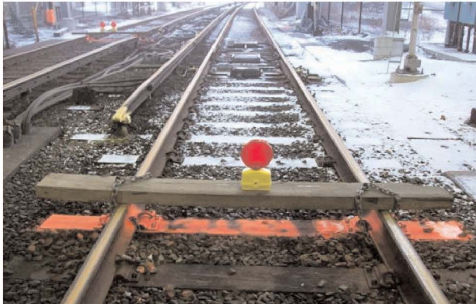
FIGURE 12 Examples of barricades. Commercially available barricade in place ( top left ); clamp-on stop flag and battery-powered red light ( top right ). Bottom photo shows work area on two-track ROW protected by barrier on each track using boards chained to rails and battery-powered red lights mounted in center of gauge ( Courtesy: MBTA ).
