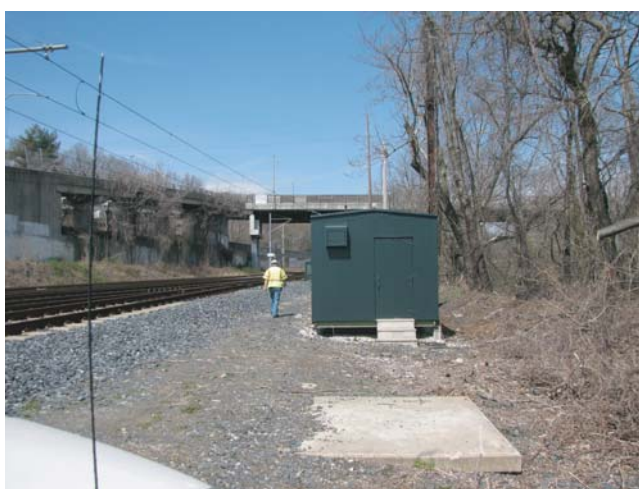
FIGURE 23 MTA interlocking signal shed and components. Speed control settings for each track within area of interlocking ( top ). MAS is maximum allowable speed for each track. Control board for interlocking within interlocking shed ( center ). Interlocking shed along the MTA ROW ( bottom ) (Photos: Chris Kozub).
