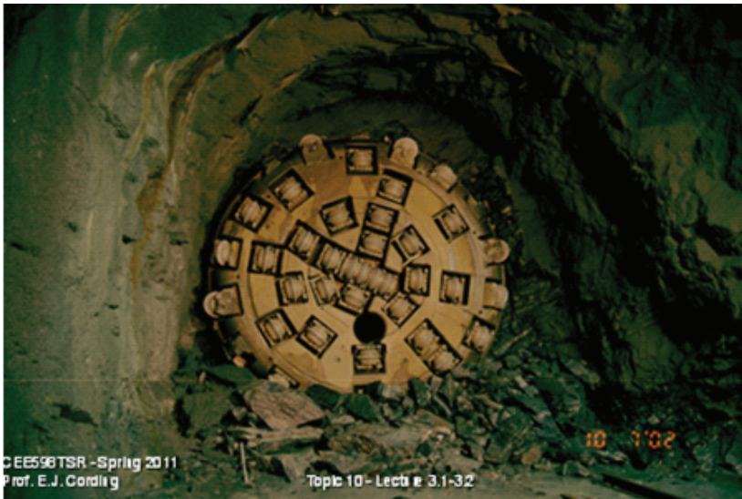
FIGURE 6.3 Cutter head of a rock tunnel boring machine used to excavate the Chat-tahoochie tunnel. Disk cutters cut grooves approximately 4 inches apart in this example. SOURCE: E.J. Cording.
