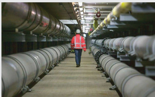
FIGURE 2 Example of a utilidor in Amsterdam that can carry multiple utility lines such as electrical, water and sewer, and communications. SOURCE: Courtesy H. Admiraal.
