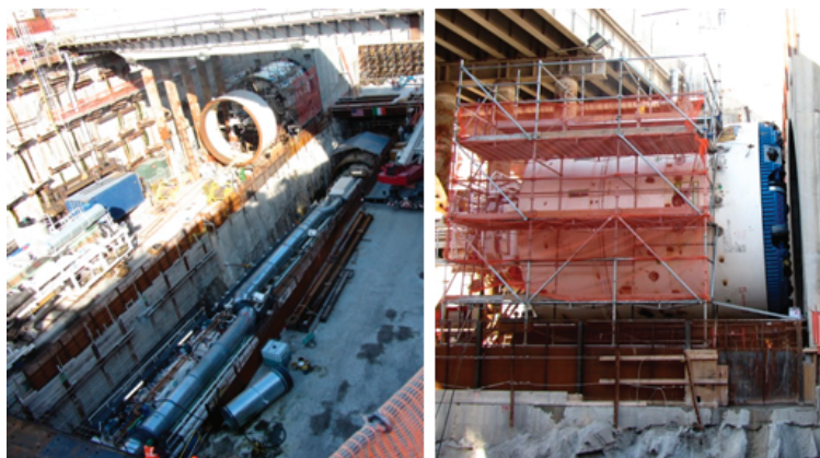
FIGURE 6.7 Slurry shield machine for the East Side Access Project, Queens, New York. (left) Assembly of two tunneling boring machines (TBM) and their trailing gear in the launch pit. (right) Closeup of the cutter head of the TBM. SOURCE: Y. Hashash.
