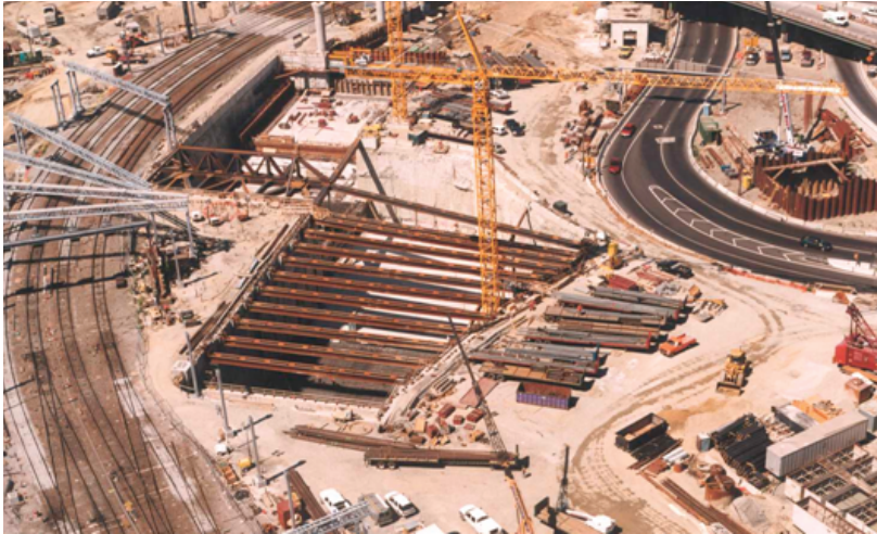
FIGURE 6.6 Braced excavation for a cut and cover tunnel section of the Boston Central Artery. SOURCE: Y. Hashash.
