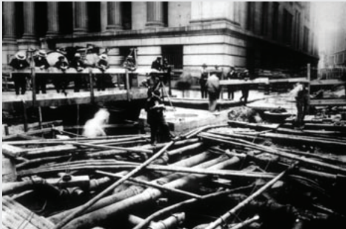
FIGURE 1 The placement of underground utility infrastructure on Wall Street (circa 1917). SOURCE: Consolidated Edison Company of New York, Inc. Reprinted with permission from Con Edison Company of New York.
