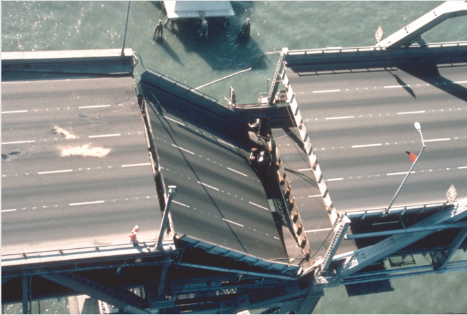
FIGURE Collapsed section of the San Francisco-Oakland Bay Bridge following the 1989 Loma Prieta Earthquake. The bridge remained closed for more than a month while the BART subway tunnel located almost directly beneath the bridge was running within a day of the earthquake. SOURCE: sanbeiji (CC-BY-SA 2.0), available at http://www.flickr.com/photos/sanbeiji/220645446/sizes/m/in/photostream/ .
