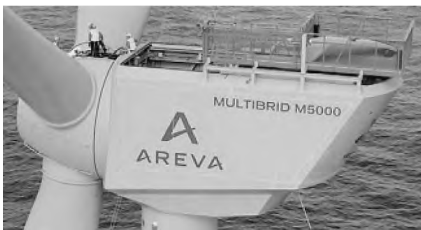
FIGURE 2-3 Offshore 5-MW wind turbine with wind technicians on board. (SOURCE: http://www.areva.com .)
