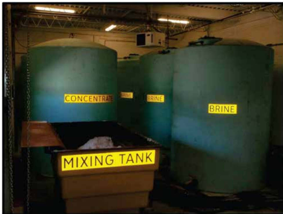
FIGURE B5 The interior of a brine making facility which houses six 5,000-gallon storage tanks, a mixing vessel that holds up to 3 tons of rock salt, and a valve control panel (Courtesy: City of Toronto).
