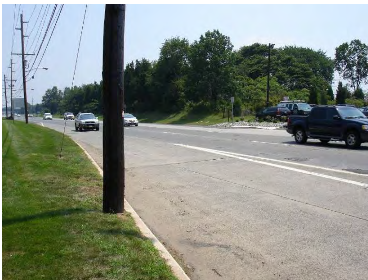
FIGURE 11 Utility poles frequently are not moved when roads are widened (New Jersey SH-22).
