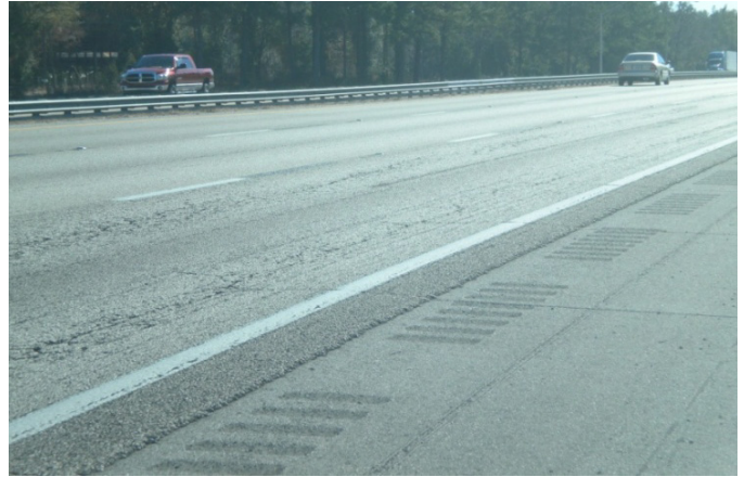
Figure 1.2. Pavement conditions between MP 413 and rest area.
