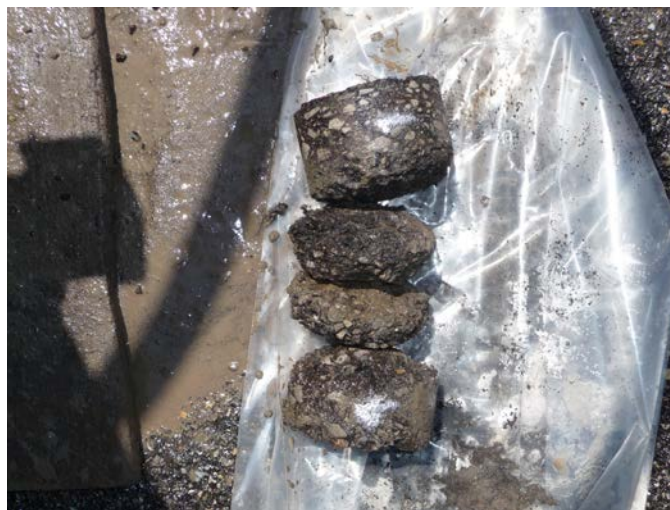
Figure 4.3. Severe stripping problems in Core 6.
