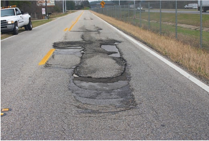
Figure 1.1. Slippage failure due to poor bond between HMA layers.
