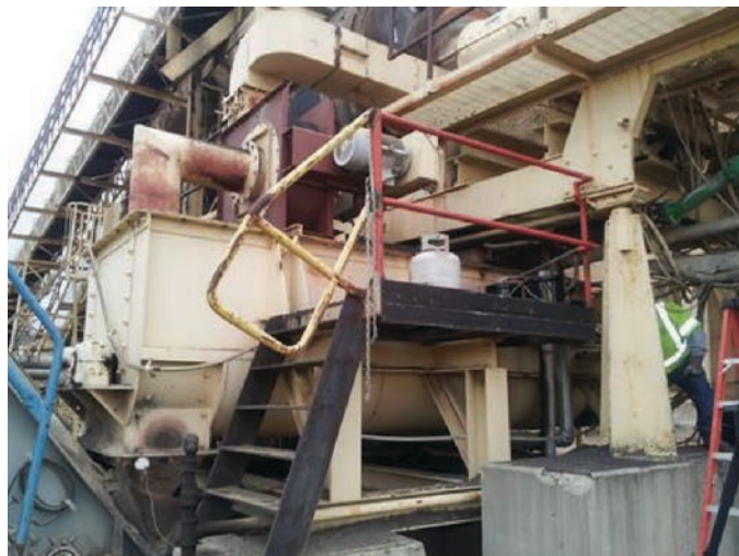
Figure 4-16. Coater box, Plant 1, Cincinnati, Ohio.
