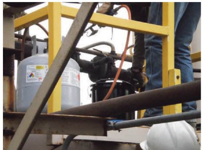
Figure 4-23. Foam sampling port, Plant 2, Fairborn, Ohio.
