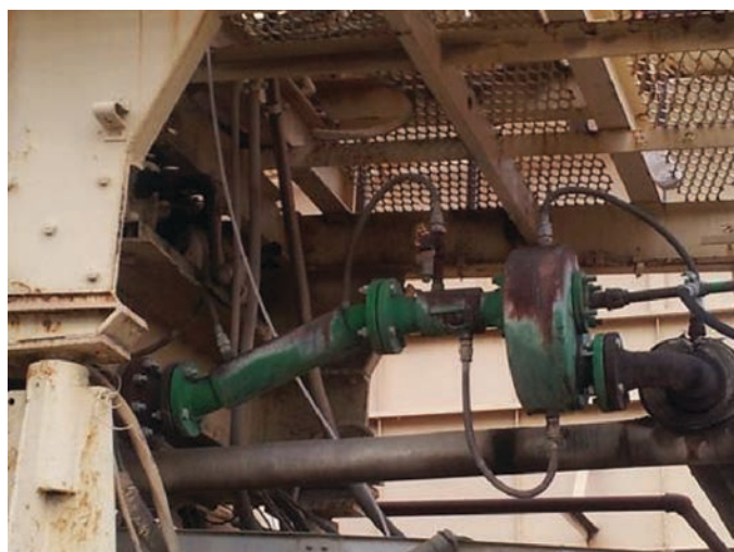
Figure 4-17. Gencor foamer, Plant 1, Cincinnati, Ohio.
