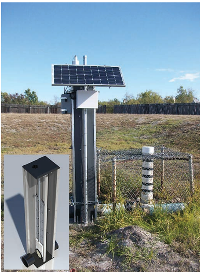
Figure 16. Active control outlet structure retrofit of dry detention basin to increase volume reduction and flow-control benefits, Pflugerville, TX. Source: Geosyntec Consultants.
