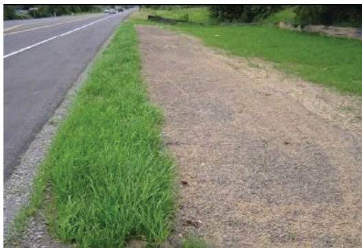
Media Filter Drain Along SR 14 in Clark County, WA. Source: Washington State DOT, 2011.
